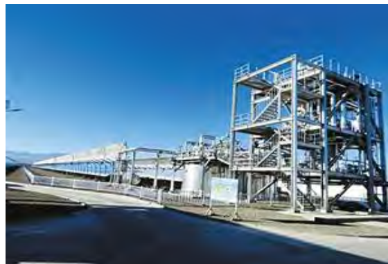
Energy storage for heat transfer area
